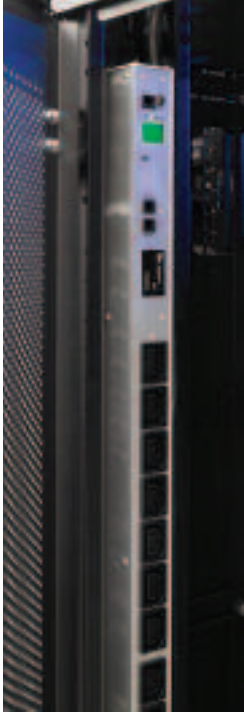
Intelligent power strips extend power monitoring to the rack.
